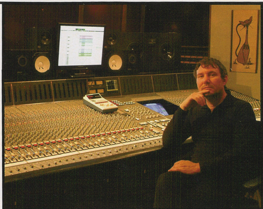
Electrokitty's Gary Reynolds claims he has installed the first commercially available Solid State Logic 9000 J Series console in the Northwest.
